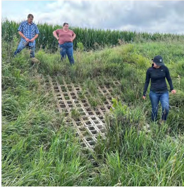
Dan Sahm, Soil Conservationist, took Mia and Gabriela to a concrete block chute site to check on it's stability.
